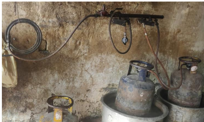
LPG Cylinders Setup to fire pit
